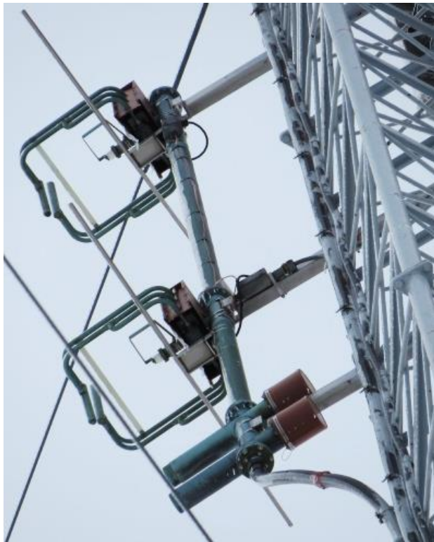
Photo by Bruce Zimmerman shows the two bay directional transmission FM antenna on the transmitter tower.
